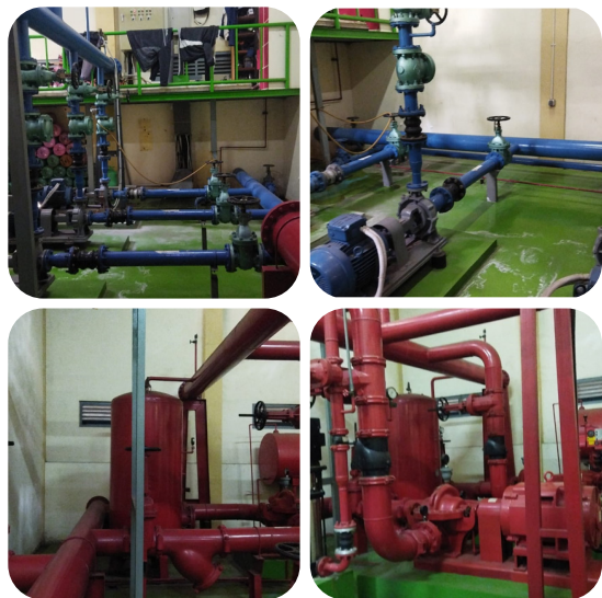
UT Water Treatment Plant
